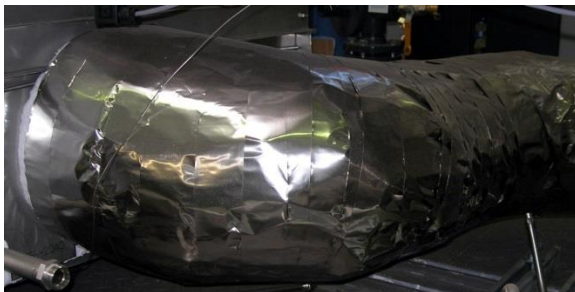
Fig. 5 Water outlet pipe with Superwool wrapped insulation
